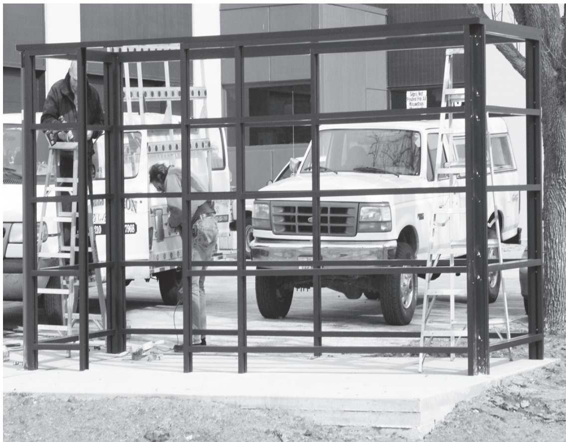
Construction workers work on the bus stop shelter in front of building 13 Nov. 2. The shelter is due to be finished by Nov. 4.
