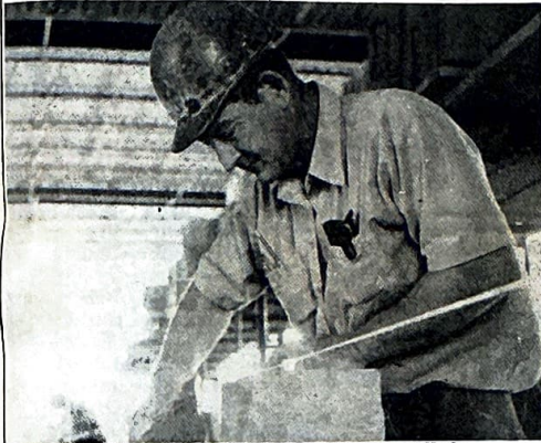
WORKMEN are presently laying interior walls in the physical plant building being constructed on the North portion of the campus.
